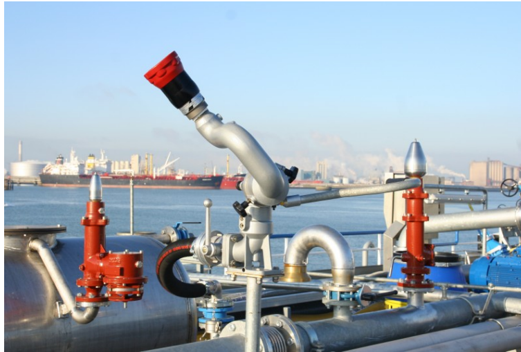
Picture: hydrant point equipped with jet/spray nozzle – with a hose of sufficient length. The somewhat “vulnerable” hose could be replaced by a fixed waterline altogether however current legislature indicates a hose is to be present.
